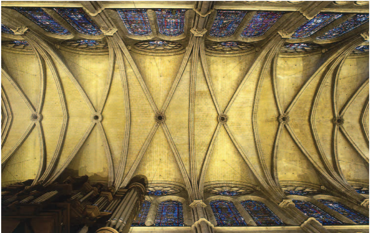
Figure 3.21. Ribbed vaults over several bays in the ceiling of a Gothic cathedral
